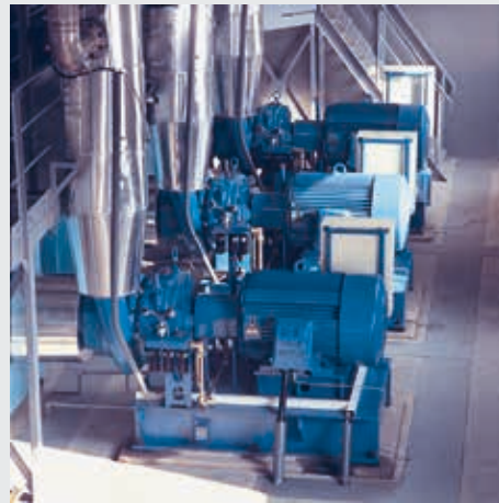
Three blowers of DA 340 type that work in Tarnów Sewage Treatment Plant; pressure rise: 60 kPa installed power: 600 kW
