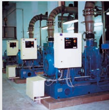
Three blowers of DA 253 type that work in Suwałki Sewage Treatment Plant; pressure rise: 60 kPa installed power: 330 kW
